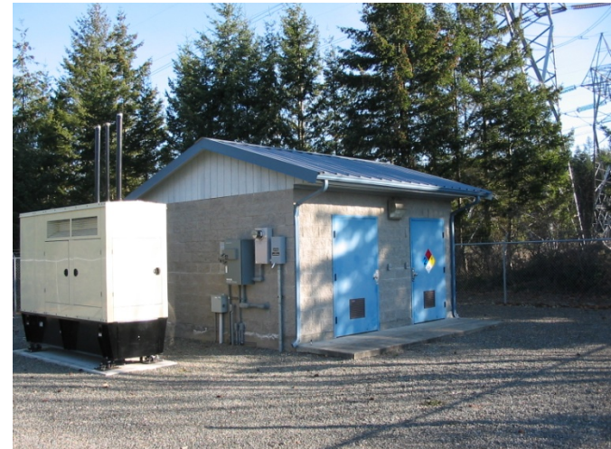
Sugarloaf Well #3 Treatment Facility
